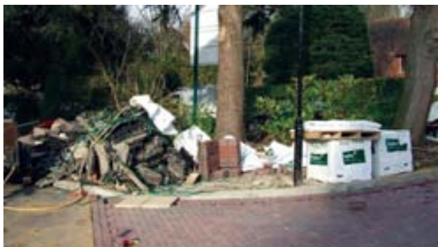
An example of bad practice. Materials are too close to the tree, restricting and damaging the roots. © Jason Hasaka / Guildford Borough Council
