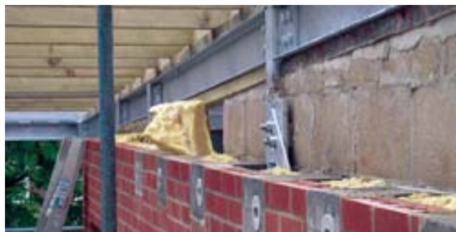
Schwegler 'swift bricks' installed under north and west facing eaves of this development in New Barnet, London © Edward Mayer / London's Swifts
