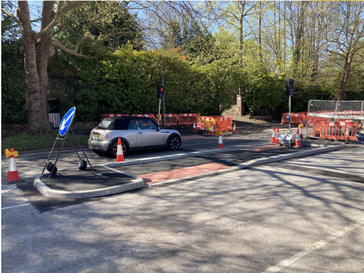
Works underway at the Epsom Road and Bushy Hill Drive junction, showing the new relocated pedestrian crossing.
