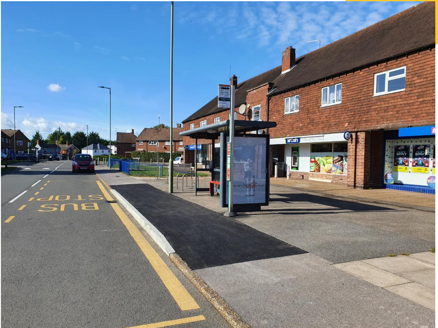
A bus stop at Stoughton Road Shops, showing completed works to install a new raised kerb and to raise and resurface the footway.
